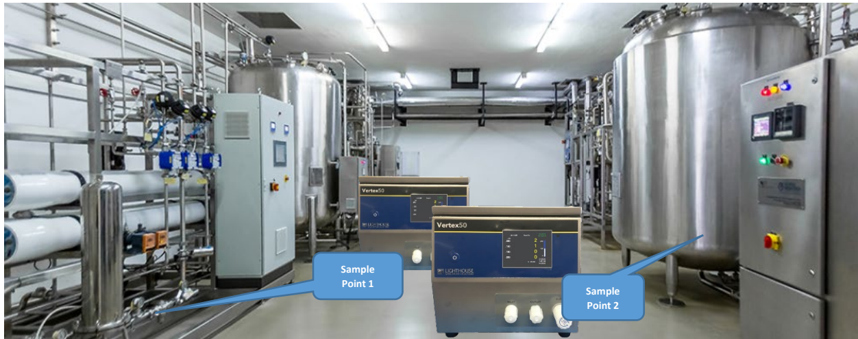
Fig 1.0 Vertex50 online monitoring of UPW system
